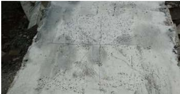
Fig. 16 Crack Pattern on Conventional Slab at the Center Span.
