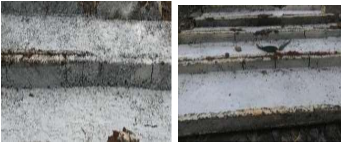
Fig.14, 15 Crack pattern on Web of Closed Channel Slab S1 and S2
