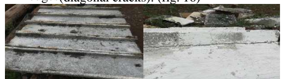
Fig. 13 Crack pattern on Web of Closed Channel Slab S1
